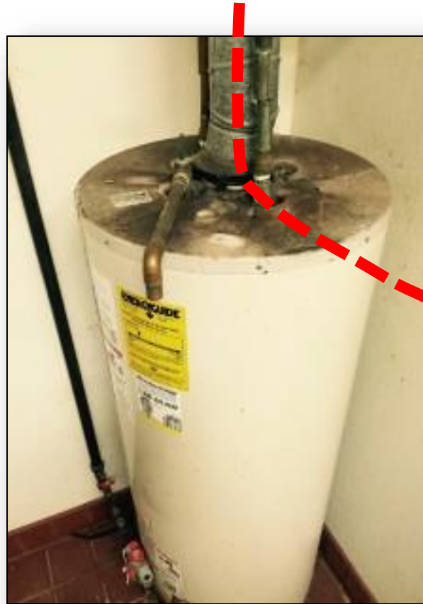
Back-drafting water heater
