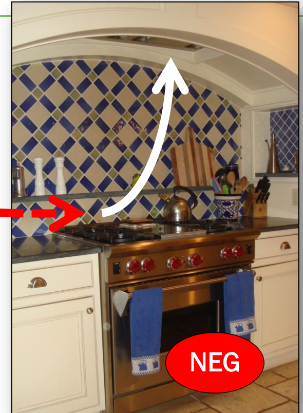
Caused by negative pressures in the kitchen
