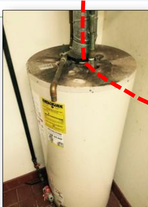
Back-drafting water heater
